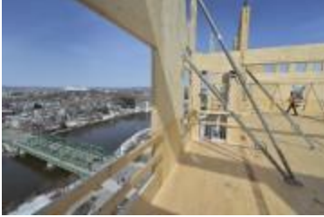
From the eighth floor, the Saint-Charles River and the Pointe-aux-Lièvres Bridge make for a beautiful northeastern panorama.
