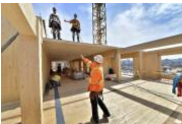
An open-air storey shows the cross-laminated timber panels and beams and the steel stability plates (on the floor).
