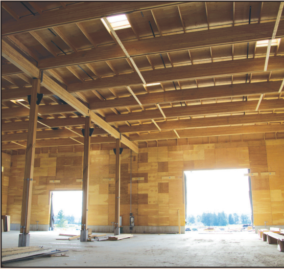
Fig. 4.9: The end walls with openings were designed as coupled shear walls, eliminating the need to provide cross-bracing for lateral resistance
