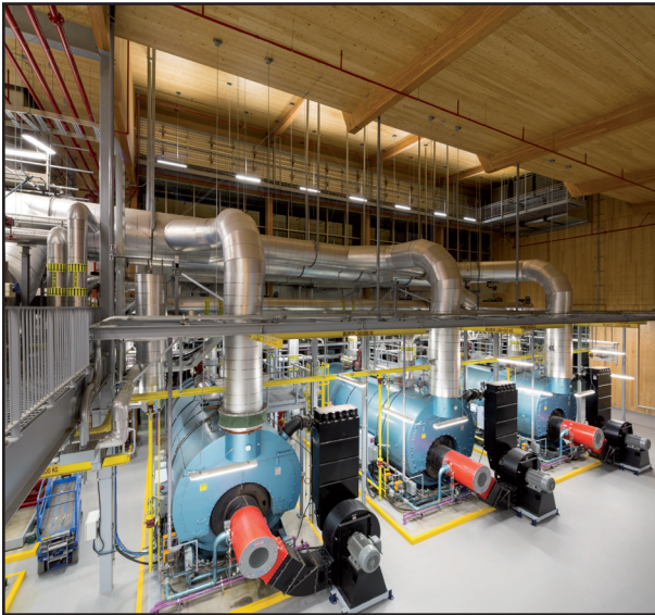
Fig. 3.4: View of boiler bay from mezzanine
