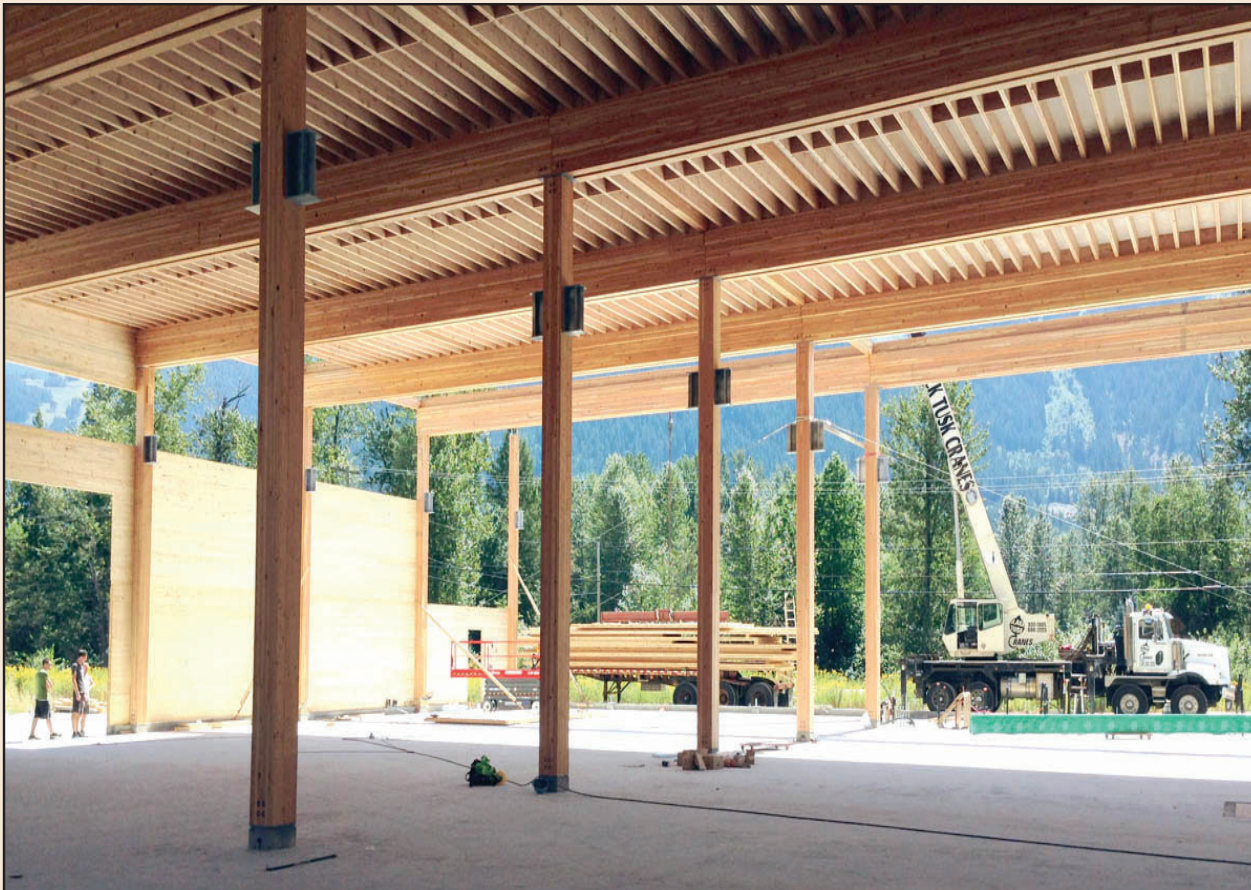
Fig. 2.9: The central line of columns reduces the depth and cost of the roof structure
