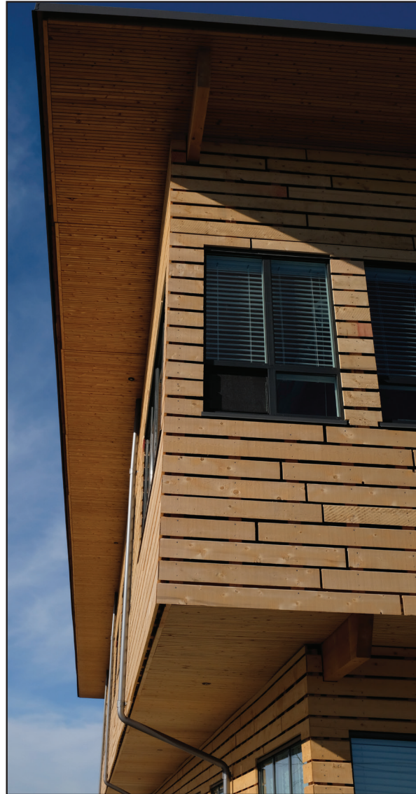
Fig. 4.16: The building is clad in a rainscreen system of unfinished Alaskan yellow cedar boards
