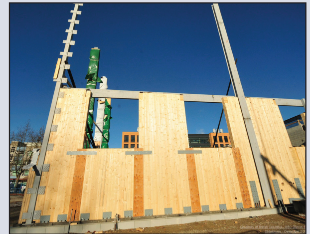
Fig. 3.9: CLT wall panels are stacked vertically and secured to the glulam frame
