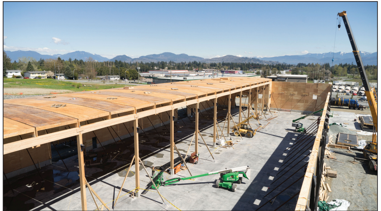
Fig. 4.10: The cambered roof beams create a sloping roof surface that facilitates drainage
