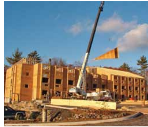
Microtel Inn & Suites, Parry Sound, ON Factory-built panelized wall systems allowed framing to be completed in 60 days without compromising quality, consistency or cost effectiveness.
