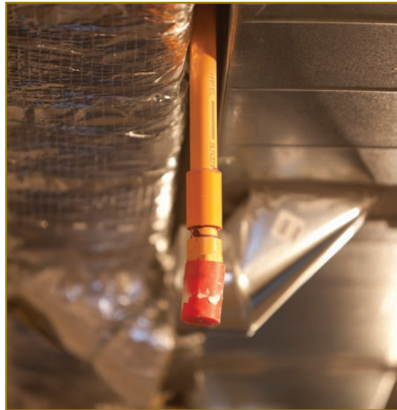
PROTECTED SPRINKLER SUSPENDED FROM CEILING
