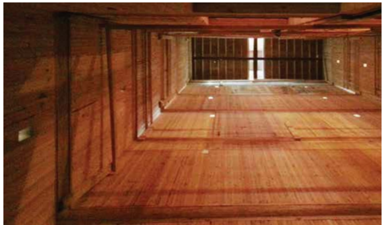
Partially constructed central stairwell (top) and elevator shaft (bottom) at Hillcrest Village, Fort St. John, B.C.
