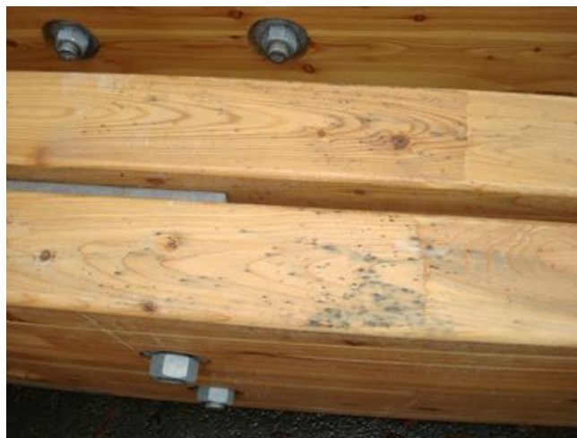
Figure 4 Iron staining on glulam resulting from on-site wetting and contamination with iron particles
