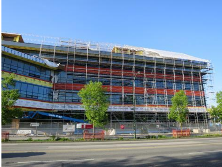
Figure 10 Using a tent to protect roof construction in a recent Vancouver project
