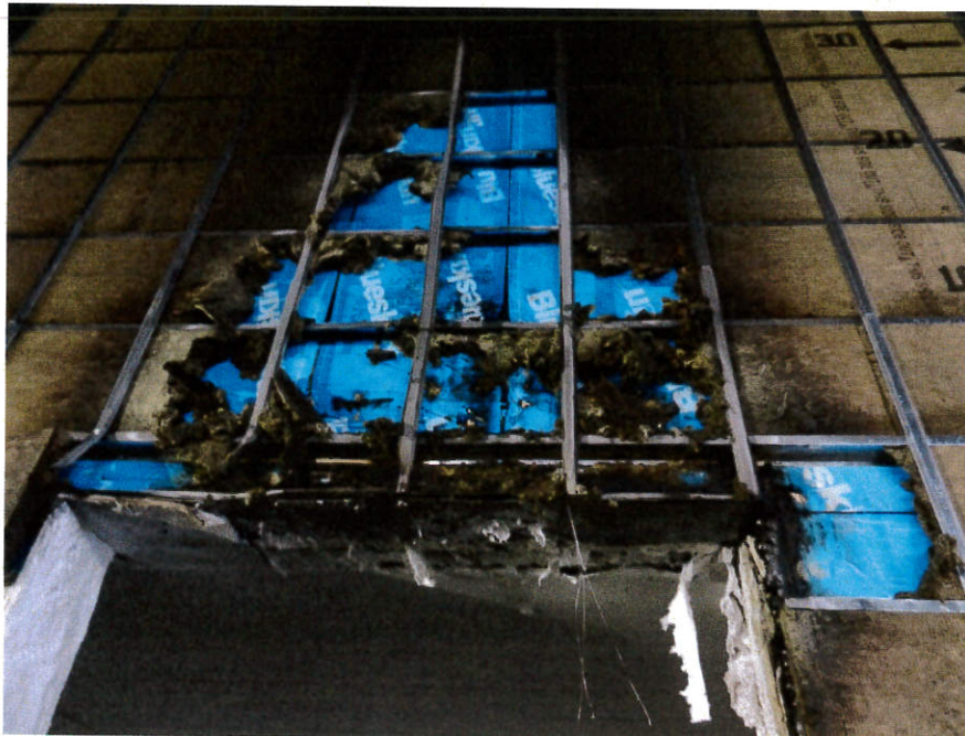
Figure 18. Insulation partially removed (showing water resistant barrier over CLT panels) after fire exposure.
