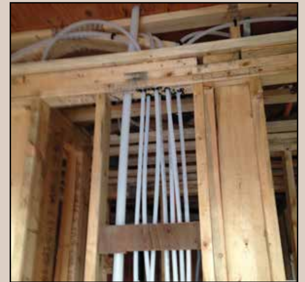
Fig. 3.12: The precision of the prefabricated frame walls enabled vertical services to be installed easily
