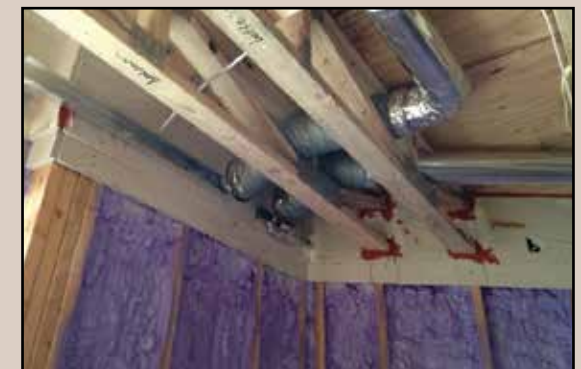
Fig. 3.5: The edges of the drywall were caulked to meet fire and acoustic requirements
