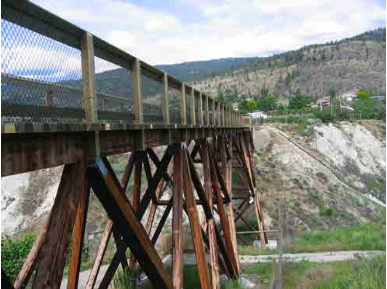
Figure 1.4.2. McCulloch Trestle foot bridge with all members sloped. (Photo Credit: D. Moses)
