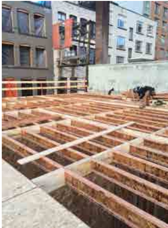
FIGURE 7.3 – SFU DOWNTOWN RESIDENCE: ALL FRAMING FOR THIS PROJECT WAS DONE ON SITE
