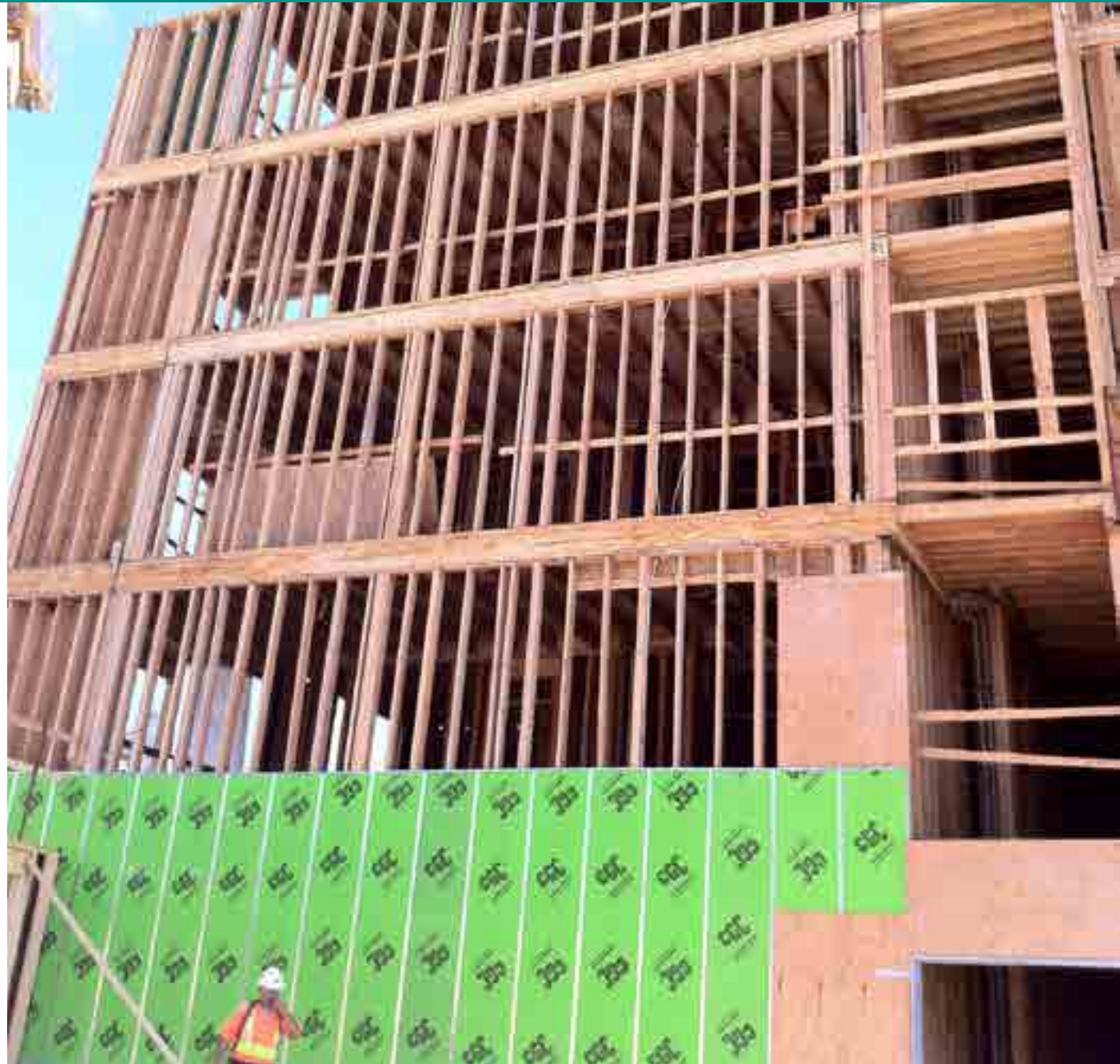
FIGURE 3.9 – SAIL: THE LOWER FLOORS USE DOUGLAS FIR STUDS FOR STRENGTH; THE UPPER FLOORS USE SPRUCE/PINE/FIR (SPF)
