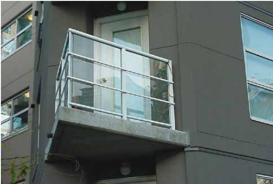
PHOTO 6: Cross cavity flashing at the floor line joint helps to return moisture to the exterior.
