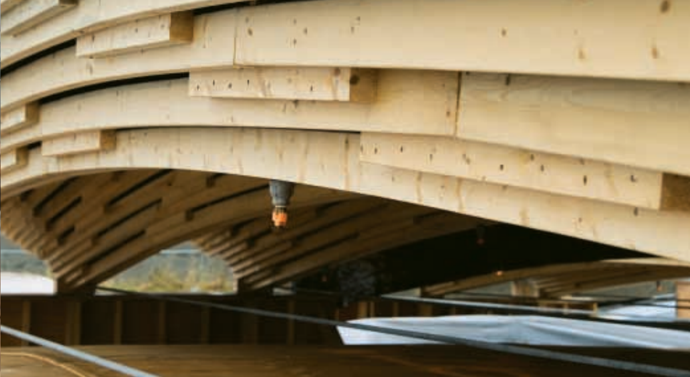
WoodWave panel - tension rods; sprinkler, wood strand pattern and form
