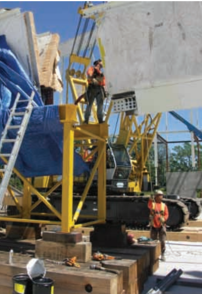
Staging of glulam arch sections on the site slab prior to the final connection of the two center span sections
