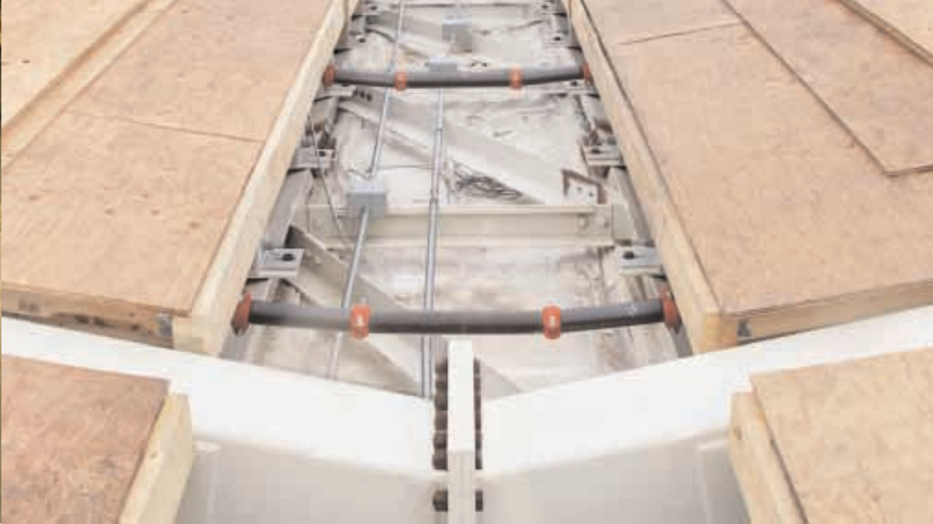
Top down roof view of an arch prior to sheathing; sprinkler system main lines, electrical conduits, ventilation system ducting, strut connection detail, WoodWave panel to arch connection detail, glulam arch steel forming and bracing elements
