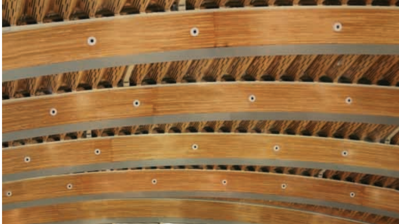
Ventilation system directional nozzles embedded in the glulam arches
