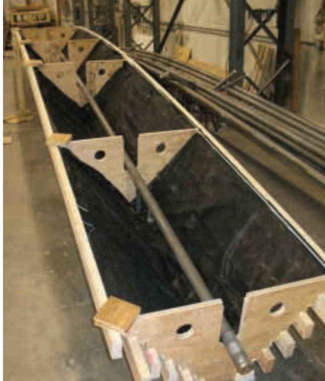
Panel Vee with sprinkler line positioned, lined with fabric and plywood gussets drilled for services
