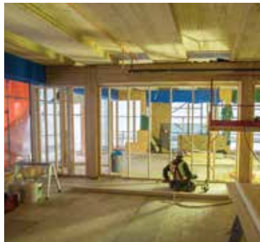
Ceiling showing the underside of overlapping CLT panels and the service chases on the floor with plywood covers in place
