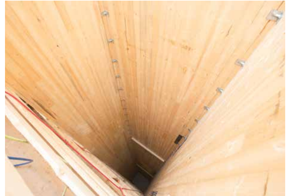
The CLT elevator shaft did not require any special acoustic treatment as it is not adjacent to noise sensitive areas
