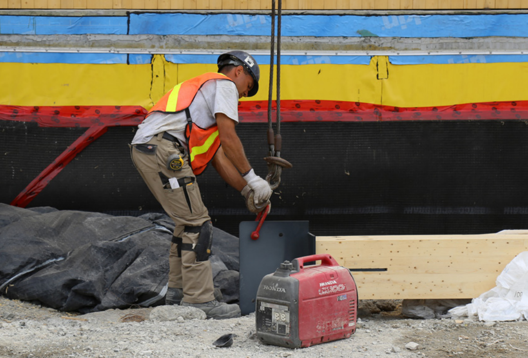
Worker attaches a glulam post to the crane in preparation for hoisting.
