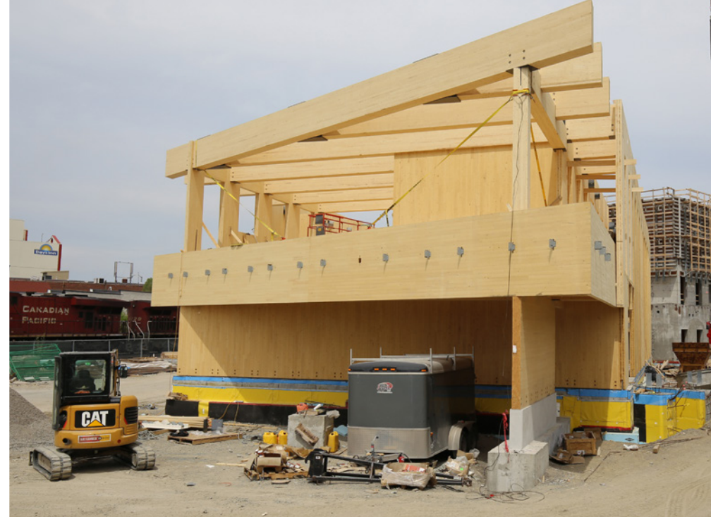
CLT structure of the library wing under construction. The entire wood structure took a small erection crew just two weeks to assemble.
