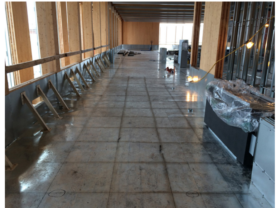
Sheet metal lines the CLT deck and kneewalls of the library's raised access floor.
