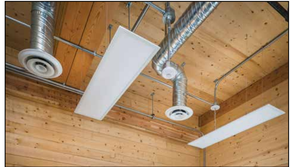
3.5 Exposed services reflect the industrial context of the building (Andrew Doran Photography, Courtesy AKA architecture + design)
