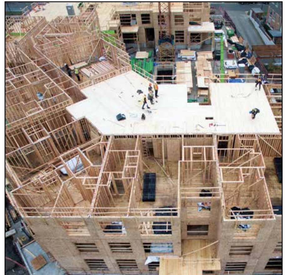
4.1 Virtuoso was the first six-storey residential building in British Columbia to combine light wood frame (for the walls) and mass timber (for the floors) construction. This technique and other all-wood approaches can now be applied to other building types. (Courtesy: Seagate Structures)
