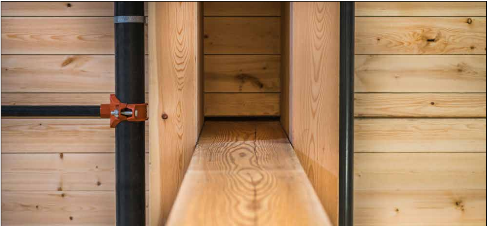
3.8 and 3.9 At mid-span, the CLT floor panels bear on a pair of glulam beams supported by a central line of glulam columns (Fast + Epp – 3.8; Andrew Doran Photography, Courtesy AKA architecture + design – 3.9)
