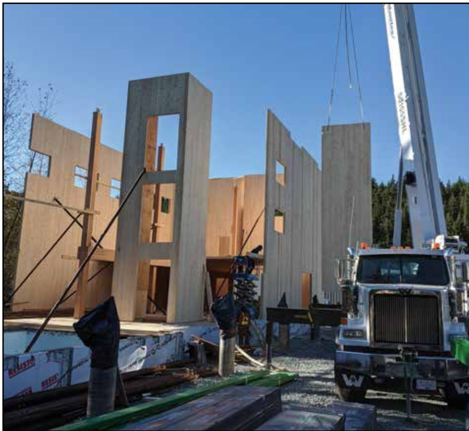
3.6 The CLT wall panels, together with the elevator and stair cores, run from grade beam to eaves as in balloon frame construction. The panels were lifted off the truck and lowered directly into place. (Fast + Epp)
