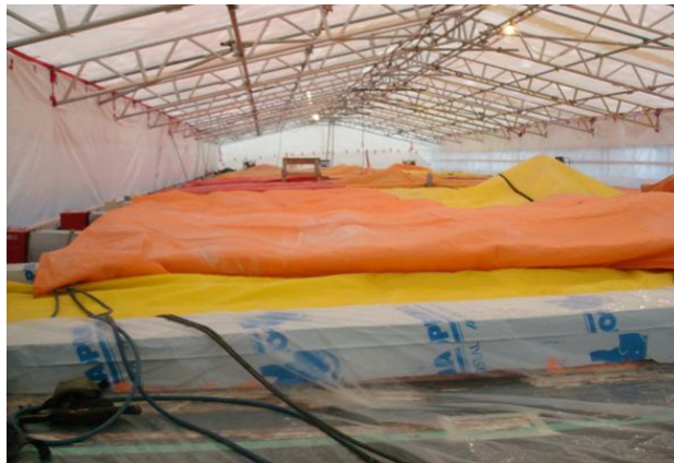
Figure 9 Drying of timber roof using electrical heating blankets under a temporary roof.
