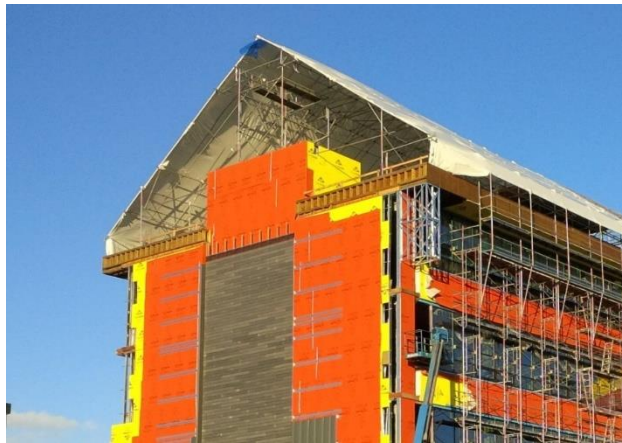
Figure 7 Using a temporary tent to protect roof construction in a Vancouver project.
