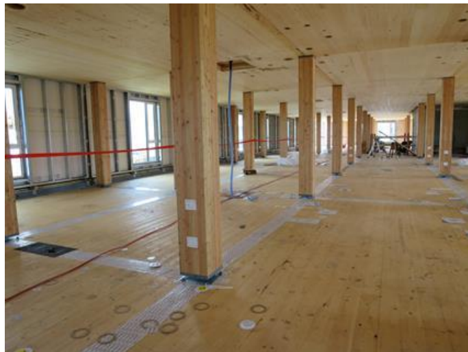
Figure 9 Joints between CLT floor panels sealed with tapes in a project in Vancouver.
