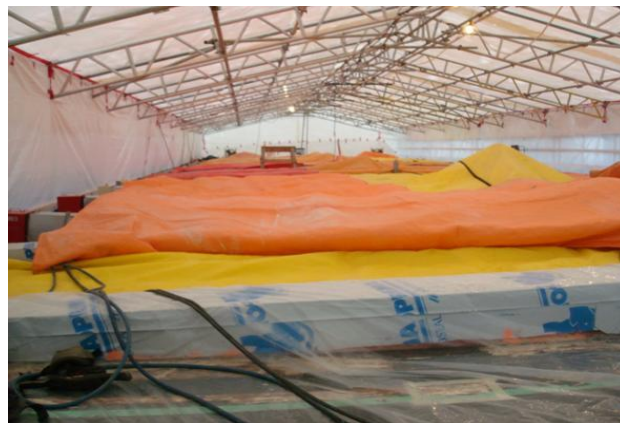
Figure 14 Drying of timber roof using electrical heating blankets under a temporary roof.
