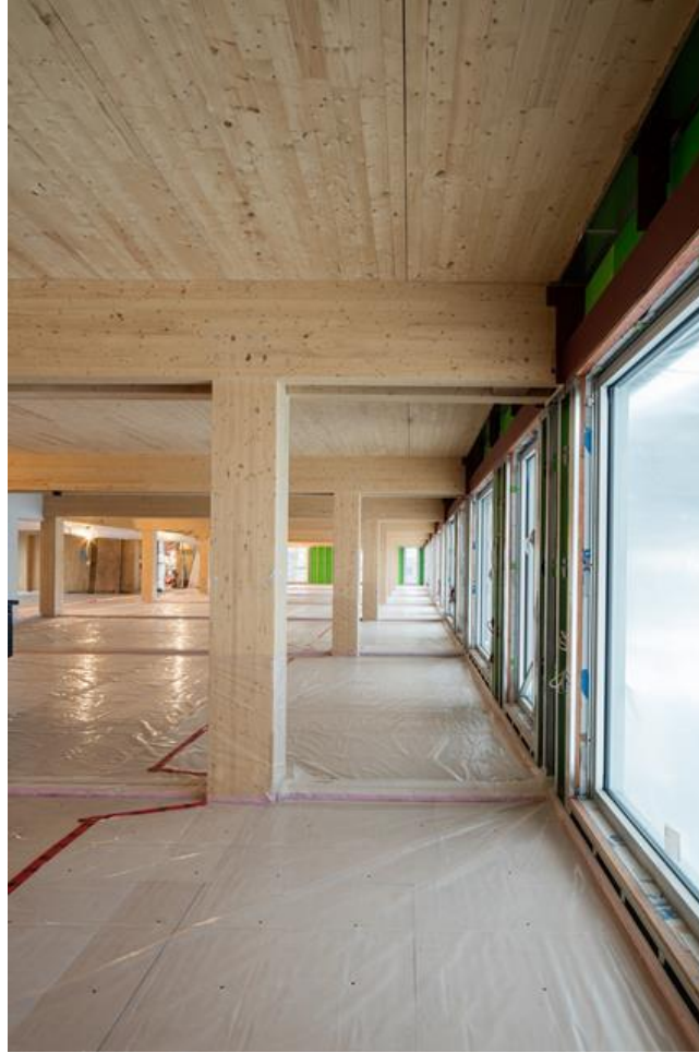
Figure 10 A floor is made watertight in a mass timber building in Montreal.
