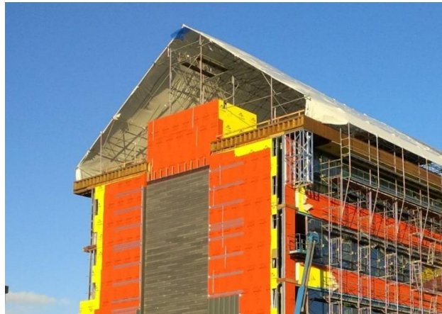
Figure 11 Using a temporary tent to protect roof construction in a Vancouver project.
