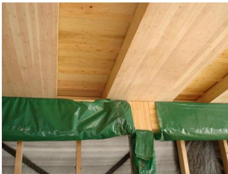
Figure 6 Interior air space built in the mass timber roof of the Wood Design and Innovation Centre in Prince George accelerating drying and enabling leak detection
