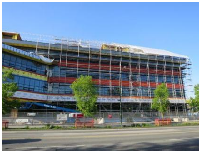
Figure 4 Using a tent to protect roof construction in a recent Vancouver project
