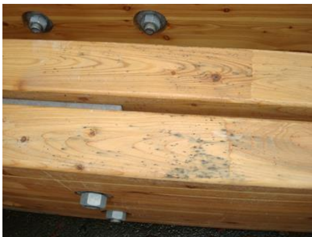
Figure 2 Iron staining on glulam resulting from on-site wetting and contamination with iron particles
