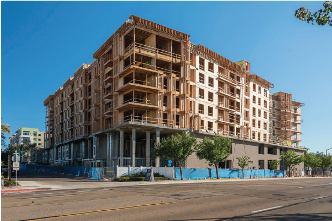
Figure 2.71: Mid-rise wood-frame building in San Diego constructing a 5-storey lightweight wood-framed structure above the 2-storey concrete podium.
