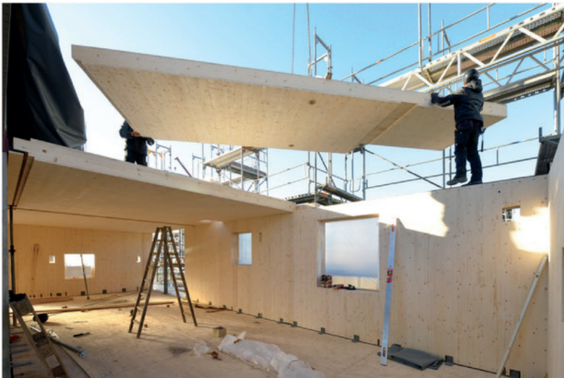
Figure 2.51: The Cube in Hamburg, Germany, is constructed using CLT panels for floor and wall structure.
