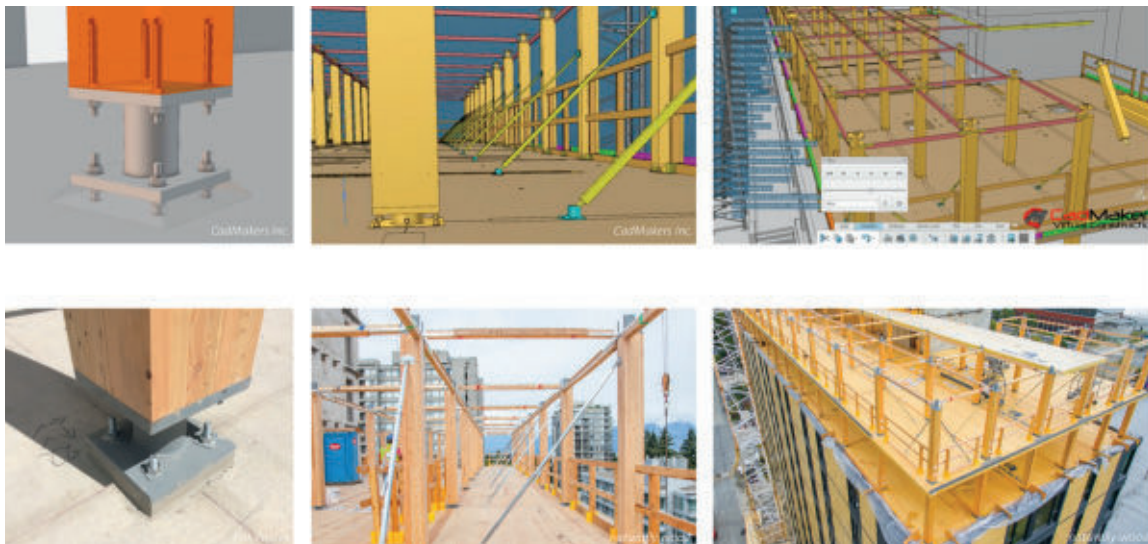
Figure 2.21: Brock Commons Tallwood House utilized various levels of Virtual Design and Construction Modelling throughout the design and construction process.
