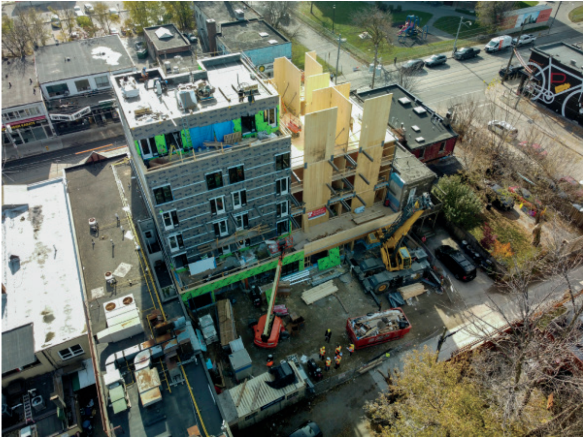
Figure 2.54: Aerial view during construction illustrating the construction staging off the rear laneway.
