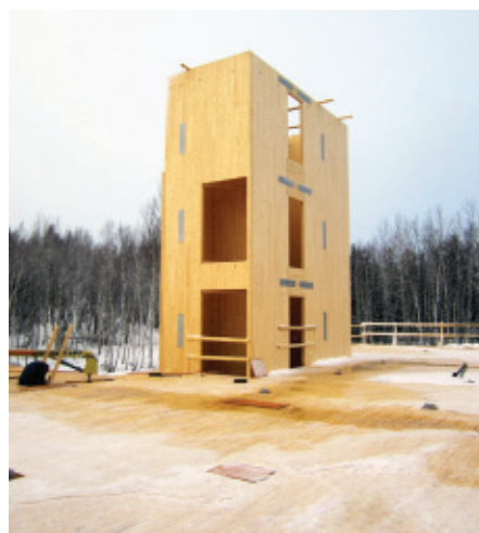
Figure 4.56: Example of an elevator hoistway composed of cross-laminated timber (CLT) solid panels.
